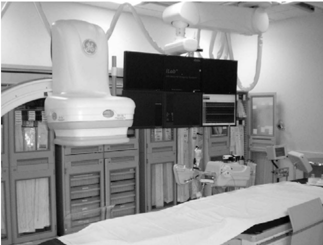
Figure 16.2. Set-up in the procedure room, with fluoroscopy machine, procedure table, screens, and infusion pumps.
